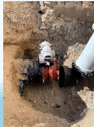
Electric actuated valve for tank fill line
