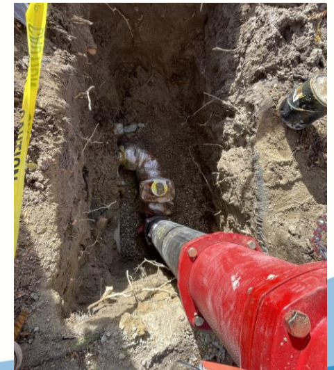
New hydrant and valve on Mock Orange Drive
