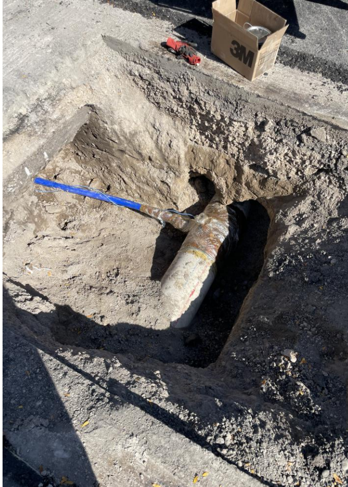
2" water lateral connection on 12" main
