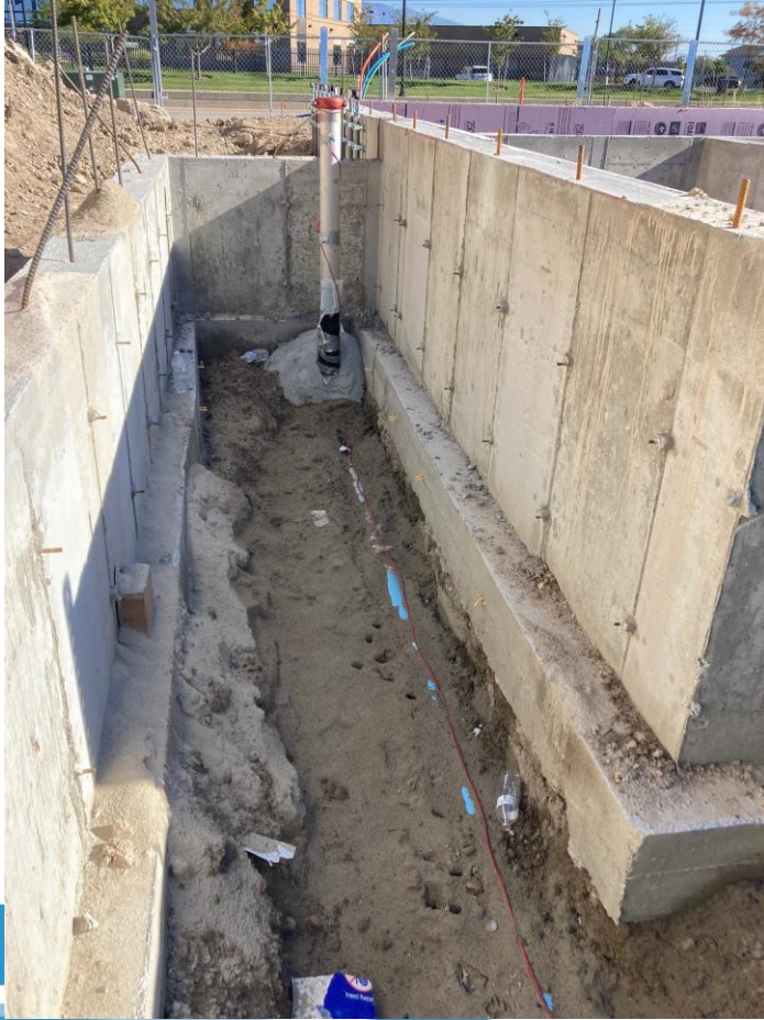
4" fire riser inside building
