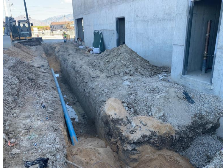
6" fire line on north side of building
