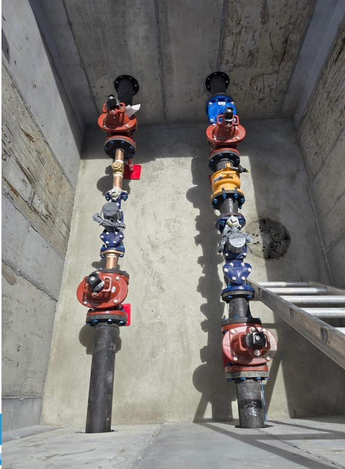
3" large meter vault
