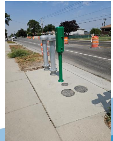
Air-vac and water sampling station vault
