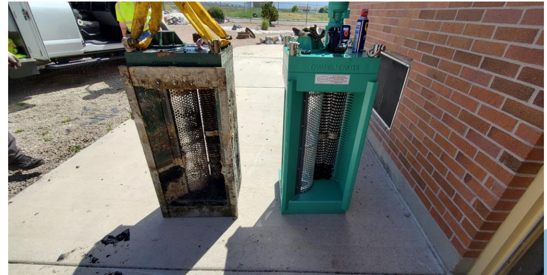
Installation at Pleasant Valley
