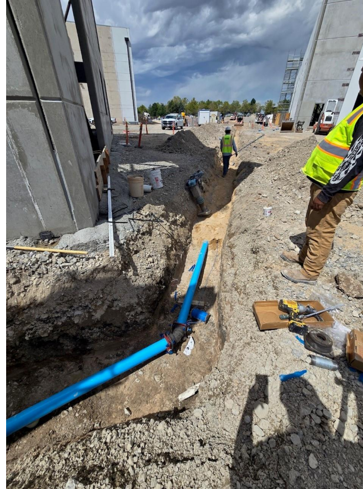
4" water lateral with fittings
