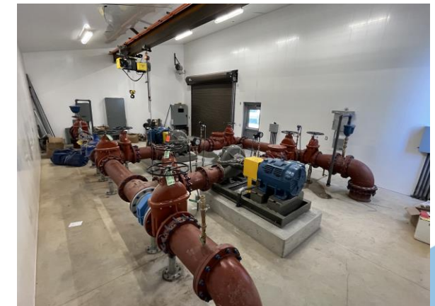
Booster Pump Station
