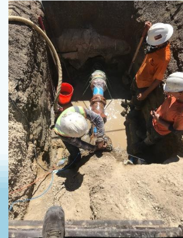
6" fireline connection with wax tape around fittings and bolts.
