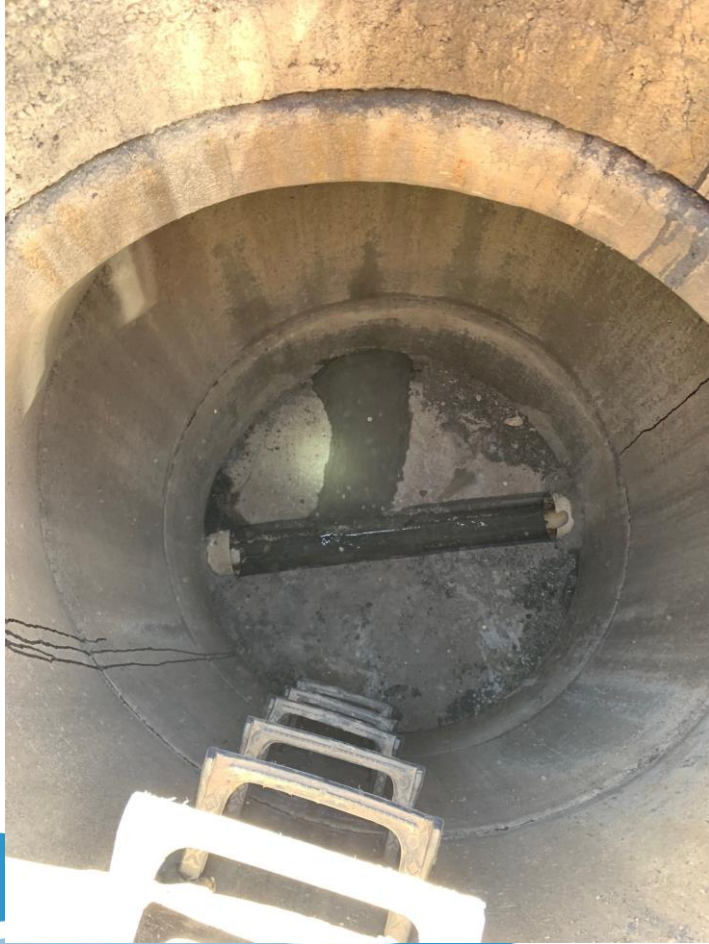
Abandoned 8" sewer - inlet trough in manhole filled with concrete
