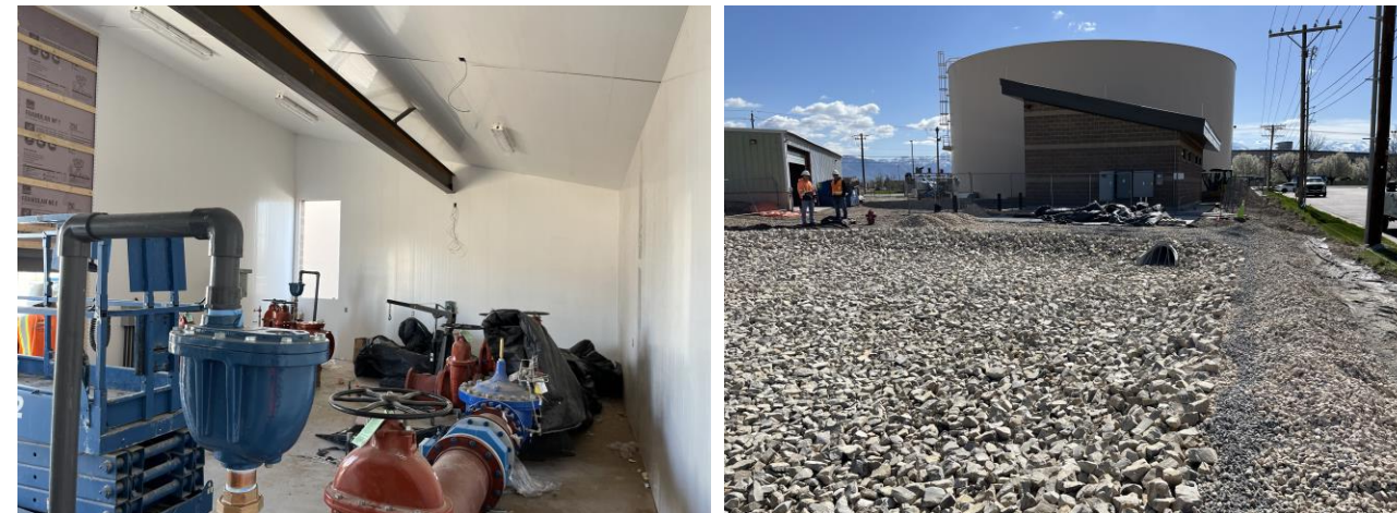
Interior and exterior photos of the booster pump station.
