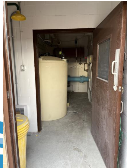
New fluoride tank installation
