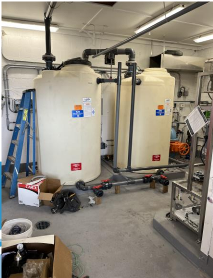
129 New chlorinator tanks and associated piping
