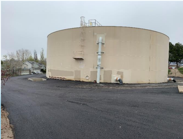
New asphalt, tank overflow piping with air gap, and safety handrails on tank roof
