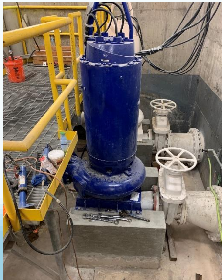
West pump installation
