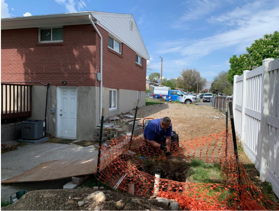
Cleanouts at northeast corner of property
