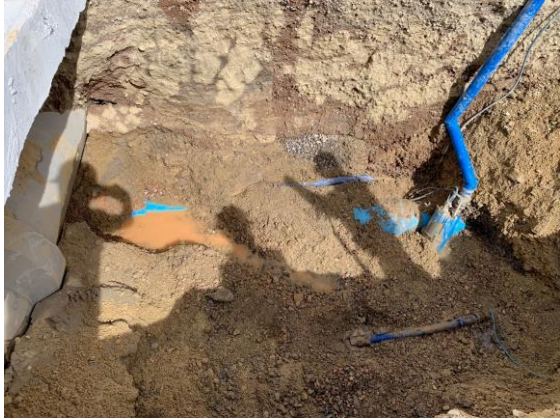
Leaking fire line
