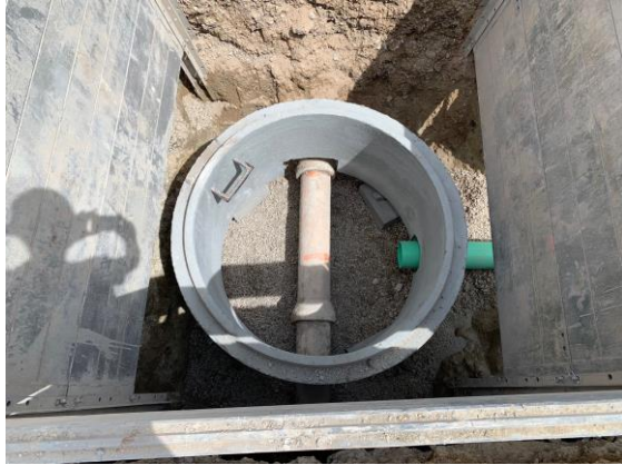
Precast manhole riser section set over existing concrete and new PVC sewer pipes
