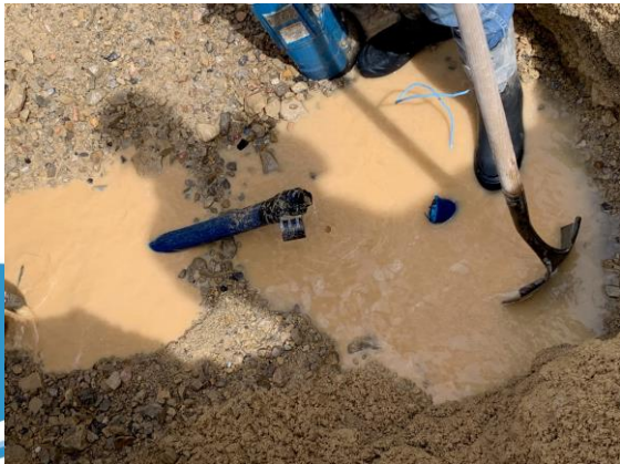
Leaking water lateral
