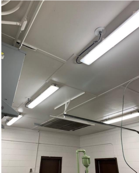
Well 12 Ceiling Paint
