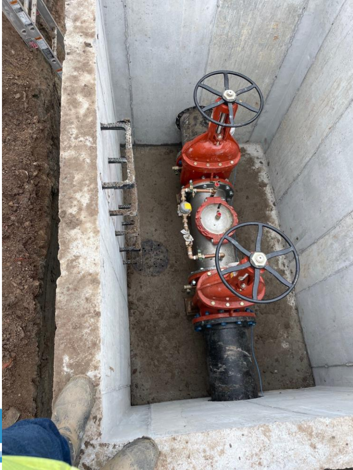
Fireline double check detector assembly in a concrete vault
