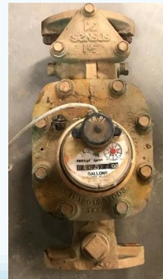
Old Turbo Meter- Not able to register in gallons
