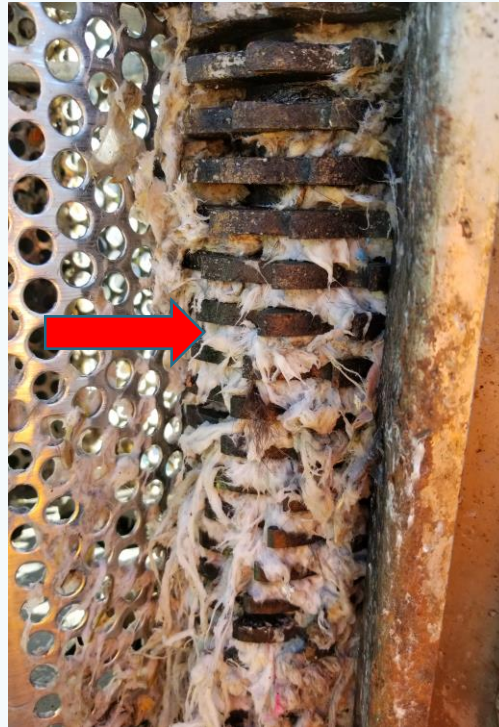
We had to use a hammer and chisel to remove the wipes from between the cutters on the Muffin Monster. You can see the wipes between the cutters.
