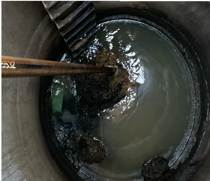
This image depicts hot asphalt that was dropped into a manhole that had hardened at Hunter Park. This happened when paving for the MVC project was performed. It was restricting flow and beginning to plug off the 18" sewer main on 3500 S.
