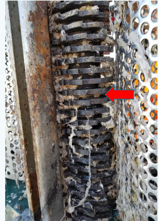
This picture shows how the Muffin Monster should look under normal conditions without the wipes between the cutters.
