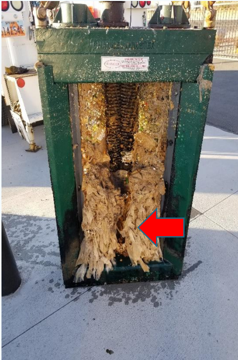
This is a Channel Grinder (Muffin Monster) we pulled in December. You can see the rags and wipes that have accumulated.
