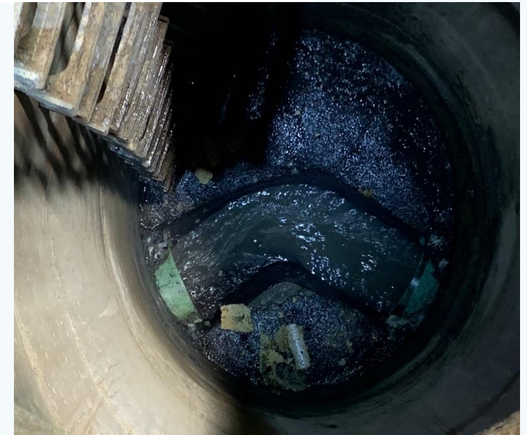
This image depicts the manhole after the asphalt was removed from the manhole and displays what it looks like under normal operation.
