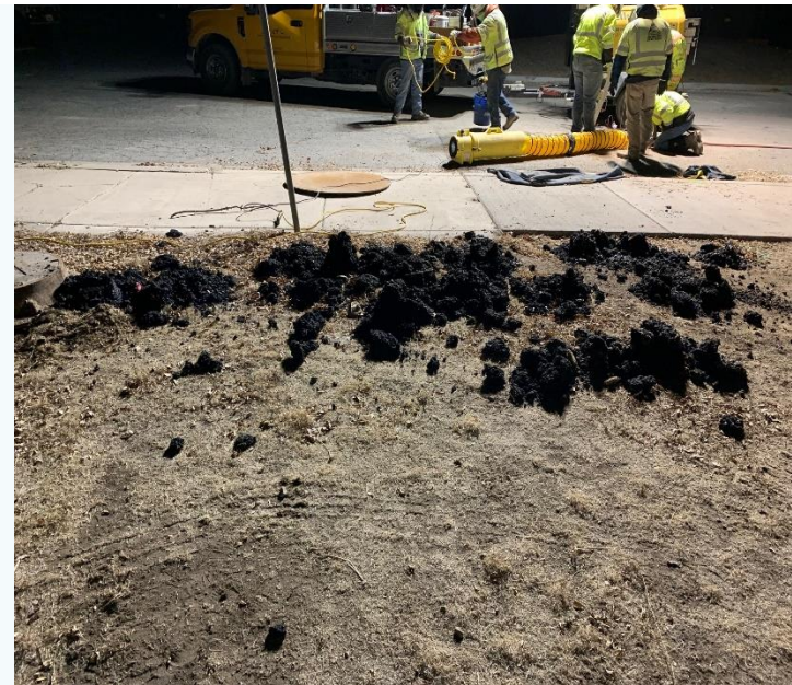
This image depicts the asphalt that was removed from the manhole at Hunter Park. The picture doesn't do much justice, but the contractor removed approximately ten 5-gallon buckets of asphalt
