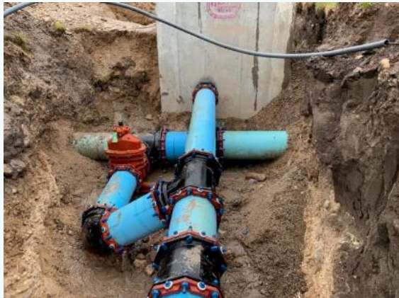
Breeze PRV Bypass
