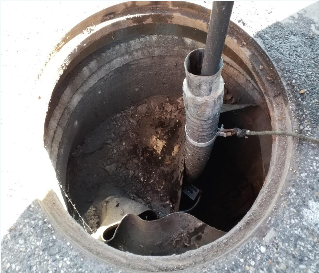
Failed Manhole Liner
