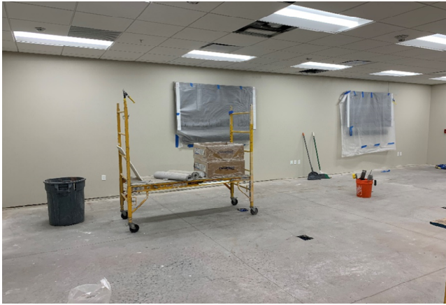
TV Installation in Conference Room
