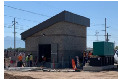
Pump station building and generator
