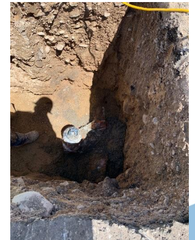
WTR to WTR connection King Valley Ln
