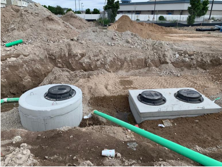
Sampling manhole and grease interceptor
