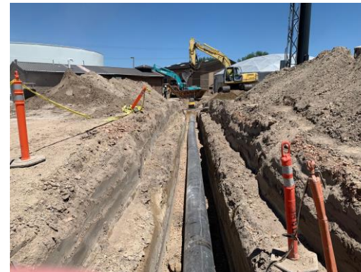
HDPE Sewer Backwash Line
