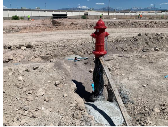
Fire hydrant with thrust block
