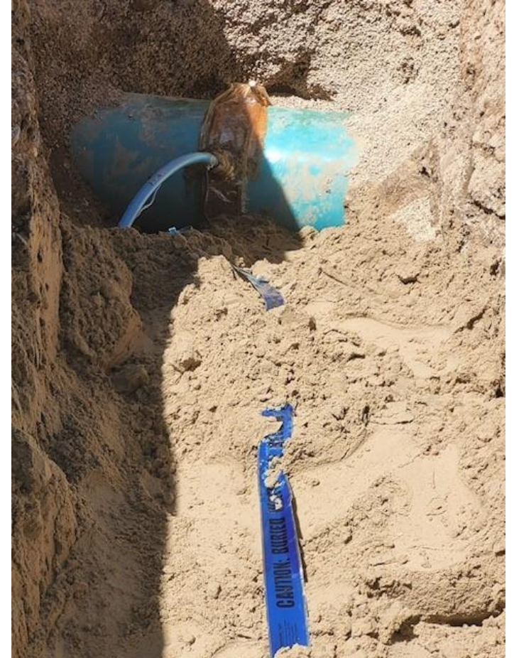
Installed water service connection
