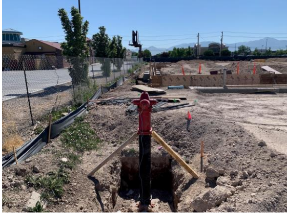
North fire hydrant
