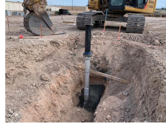
6" fire riser with thrust block
