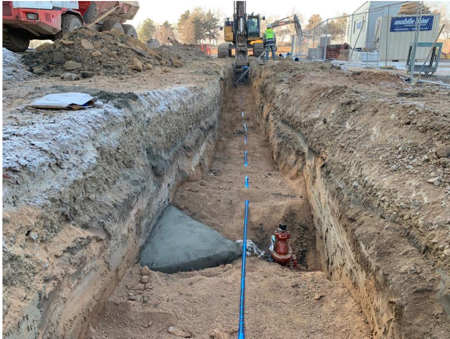
8" fire line trench with compacted bedding, warning tape, and thrust block for valve
