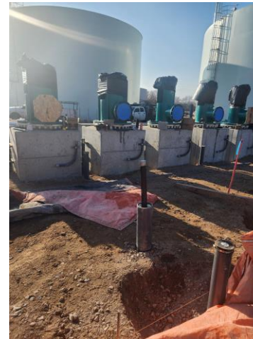
View of installed pumps
