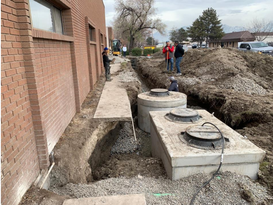
View of grease interceptor and sample manhole
