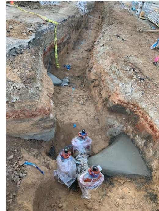
Thrust block for valve cluster
