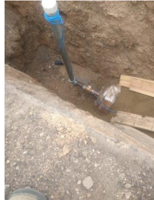
Blow-off on West end of line
