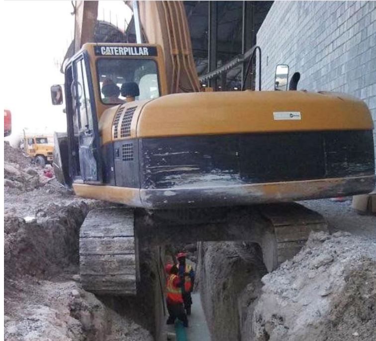
Hazardous Trench – stock photo.
