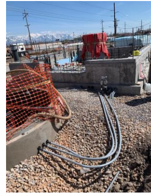
Electrical conduits from wet well to electrical building
