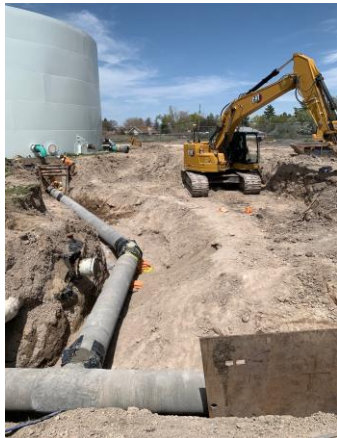
Outlet piping - 24" cement-mortar lined steel piping for 1MG and 2 MG tanks
