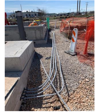
Electrical conduits from pig launch vault to electrical building
