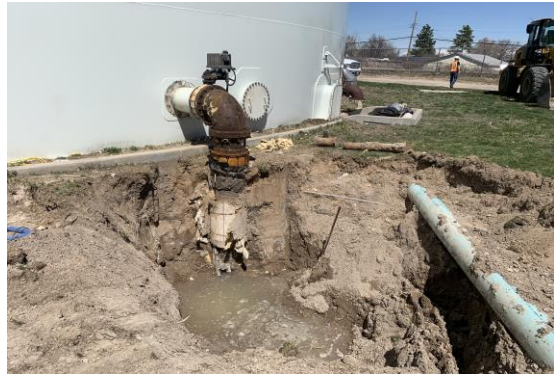
Exposed piping near 2 MG tank
