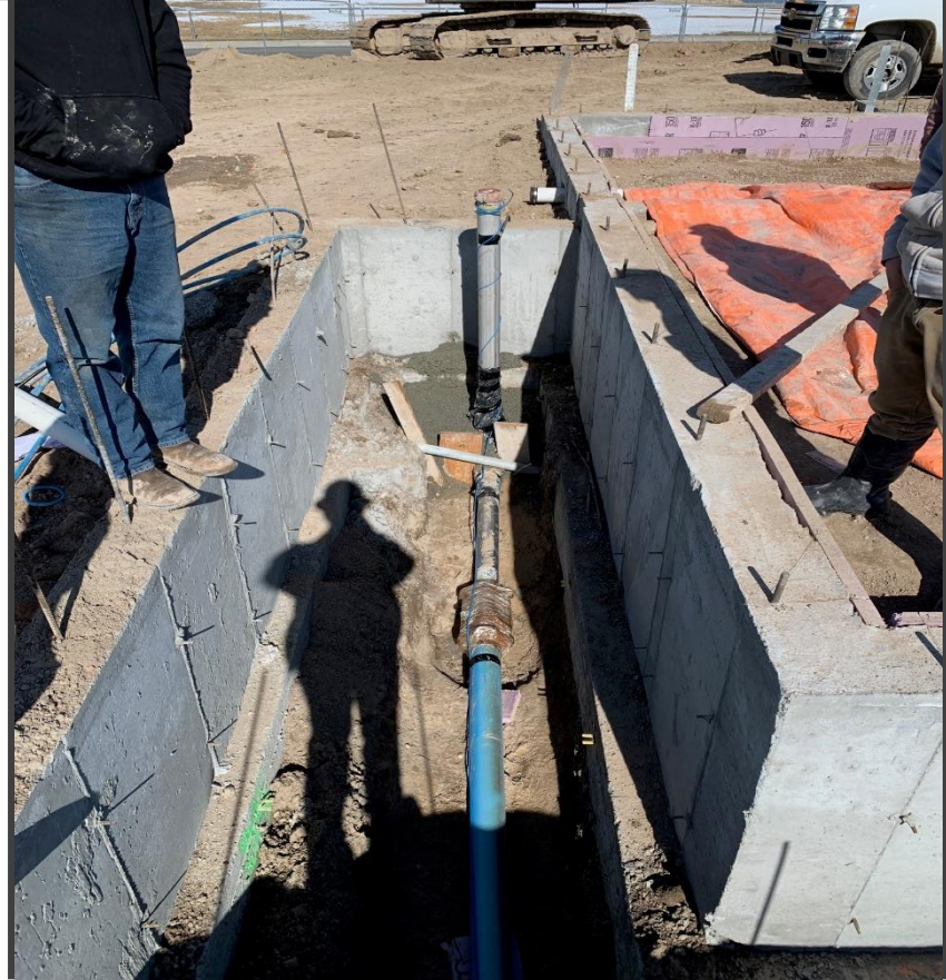
Fire riser with thrust blocking
