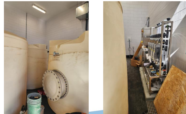
Chlorine room with tanks and chlorine generator
