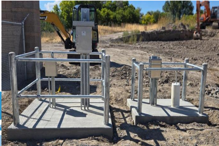
New Cathodic Protection Anode Well and Control Panel
