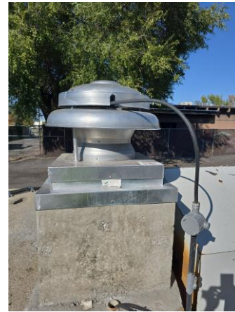
Wet Well Exhaust Fan on New Concrete Housekeeping Pad
