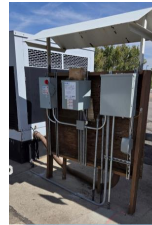
New Electrical Panel, Transformer, and Disconnect
