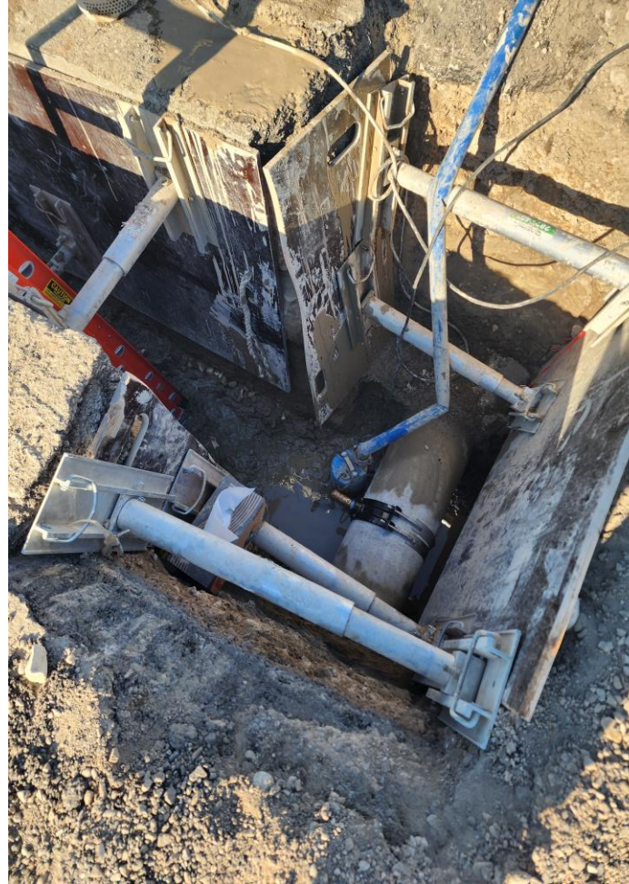
3/4" tapping saddle on GHID 12" asbestos cement water main
