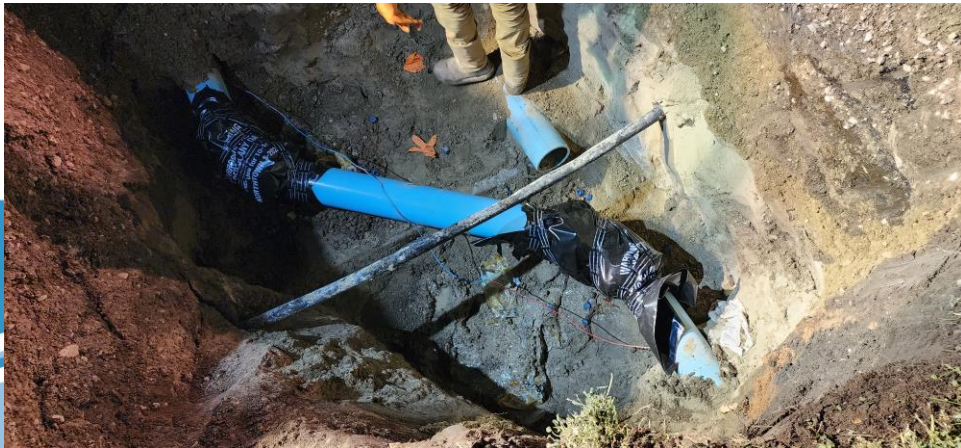
Fire Line Connection
