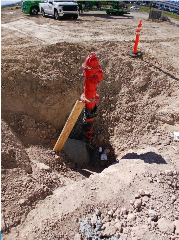
Fire hydrant with thrust block
