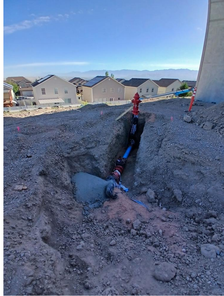
Fire hydrant, valve, and thrust block
