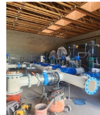
Pump motors and discharge piping
