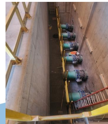
Pump suction piping
