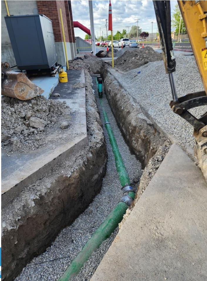
Ductile iron epoxy coated 8" sewer pipe
