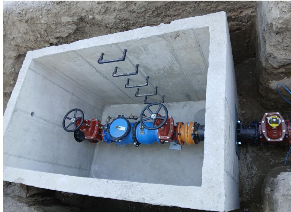
8" Double Check Detector Assembly (DCDA) Vault
