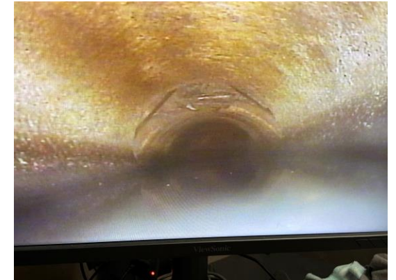
Joint offset in pipe
