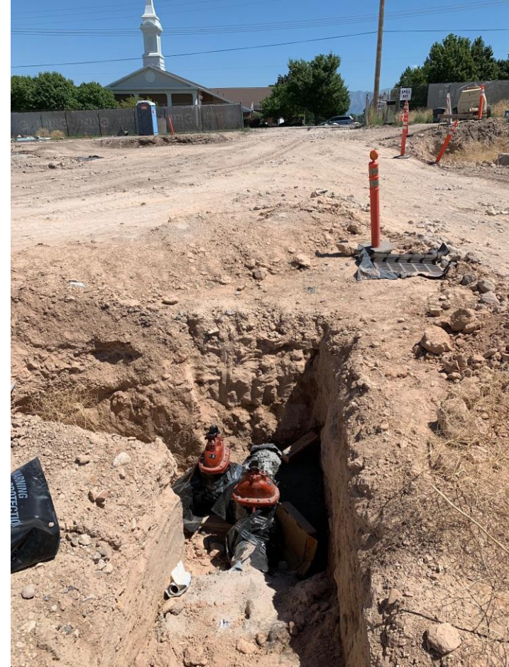
Southeast fire line tee and valves
