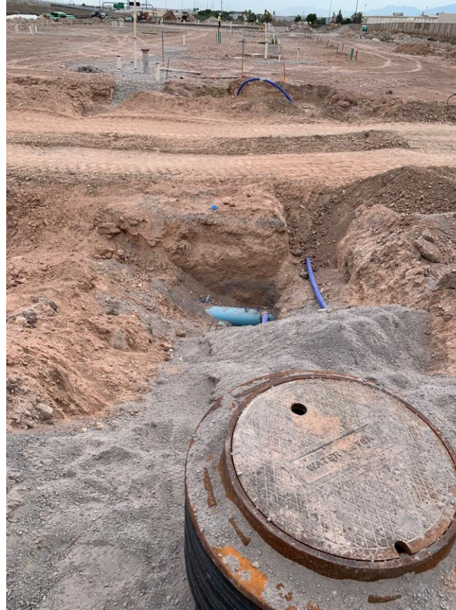
2" meter on south side of new building
