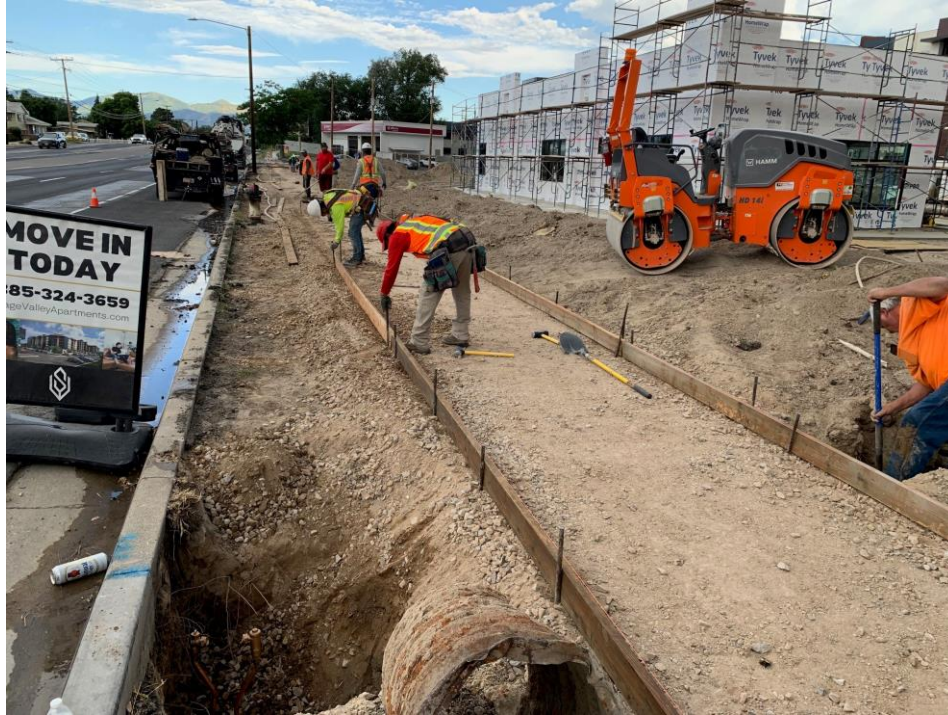
\frac{3}{4} " landscape meter setter behind curb
