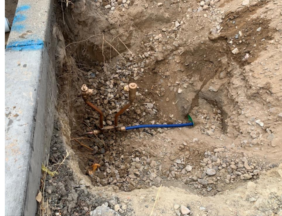
\frac{3}{4} " landscape meter setter and poly pipe lateral
